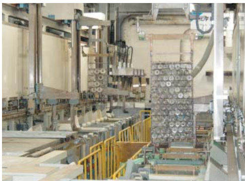
Automatic chemical surface treatment
